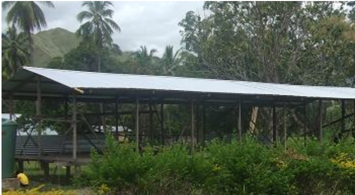
Left: Incomplete classrooms
